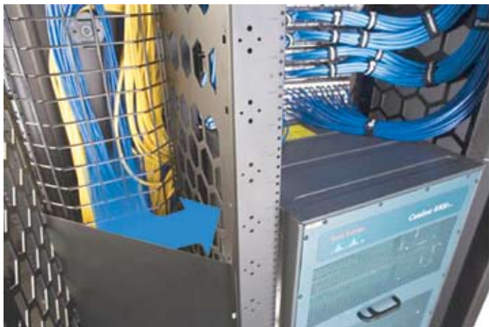
Figure 4. Baffles and perforations can maintain front-to-back airflow in racks containing side-ventilated equipment.
